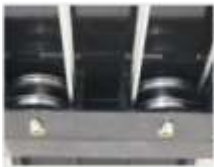
Cable and pulley under main platform.
