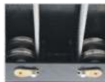
Cable and pulley under main platform.
