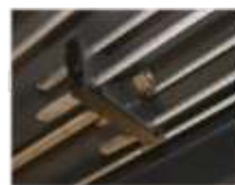
Cable connection under main platform.
