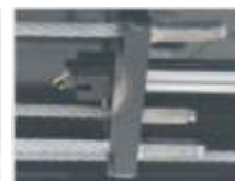
Cable connection under main platform.
