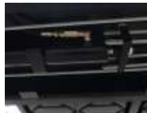
Hydraulic cylinder under runway with explosion-proof valve.
