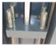
Cable connection under main platform.
