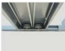
Cable and pulley under main runway.
