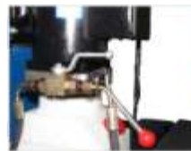
The valve control platform and rolling jack.
