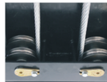
Cable and pulley under main platform.
