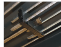
Cable connection under main platform.
