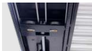
Pulley and cable under upper main platform
